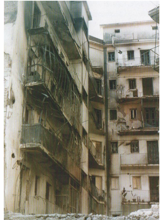
Damage by fire on a reinforced concrete building (Pucinotti, 2005)
