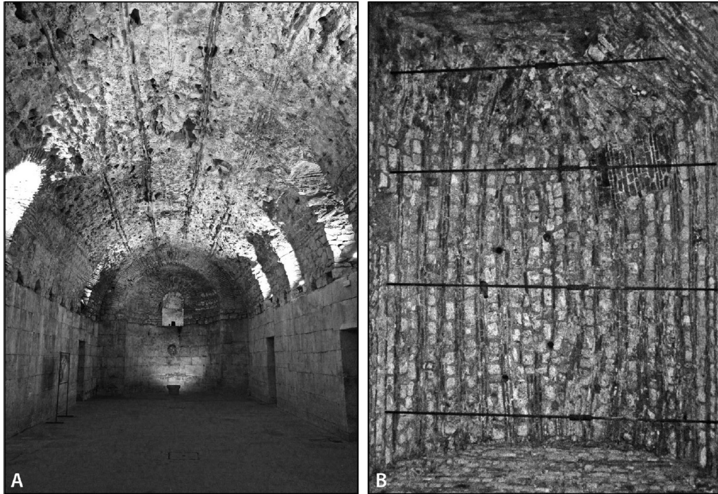
13. Examples of radially laid caementa combined with courses of radially laid brick. A: Substructures of the Palace of Diocletian at Split, Croatia (early fourth century CE). B: Praefurnium for caldarium of the Imperial Thermae at Trier, Germany (early fourth century CE). Note vertical tubes in vault for ventilation. The iron tie bars are modern. (Color image: WebFig. 6).
