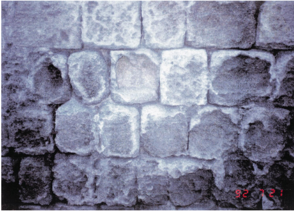
Figure 7. Incompatible modern cement restoration mortars trigger intense corrosion of the porous building stones by salt decay. Detail of the masonry near the Sea Gate of the fortifications.
