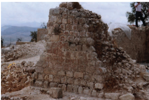
Fig. 8. Ruins of the Castle of Cañete la Real (Malaga, Spain). The piece of wall shows extensive loss of joint mortar linking the stone blocks.
