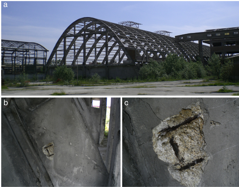
Fig. 1. a) Ex-Agrimont industrial plant, C3 building; b, c) concrete degradation on an arch in the south-western section of the structure.
