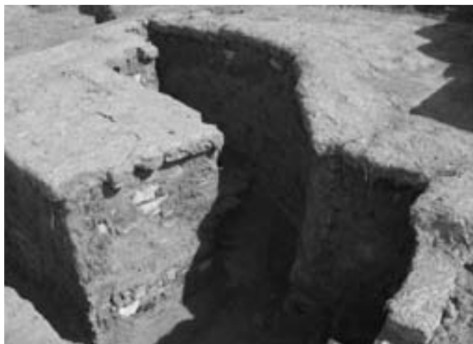
FIGURE 4 The raising of brick walls covered with adobe plaster as a means of protecting the main walls. Photo: Manijeh Hadian, RCCCR
