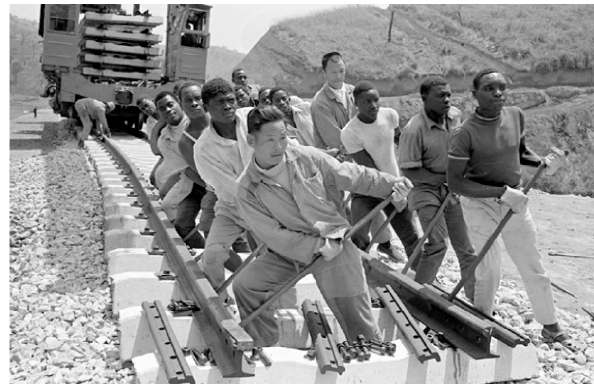
Figure 4. Chinese and African laborers work at the construction site of the TAZARA railway.
